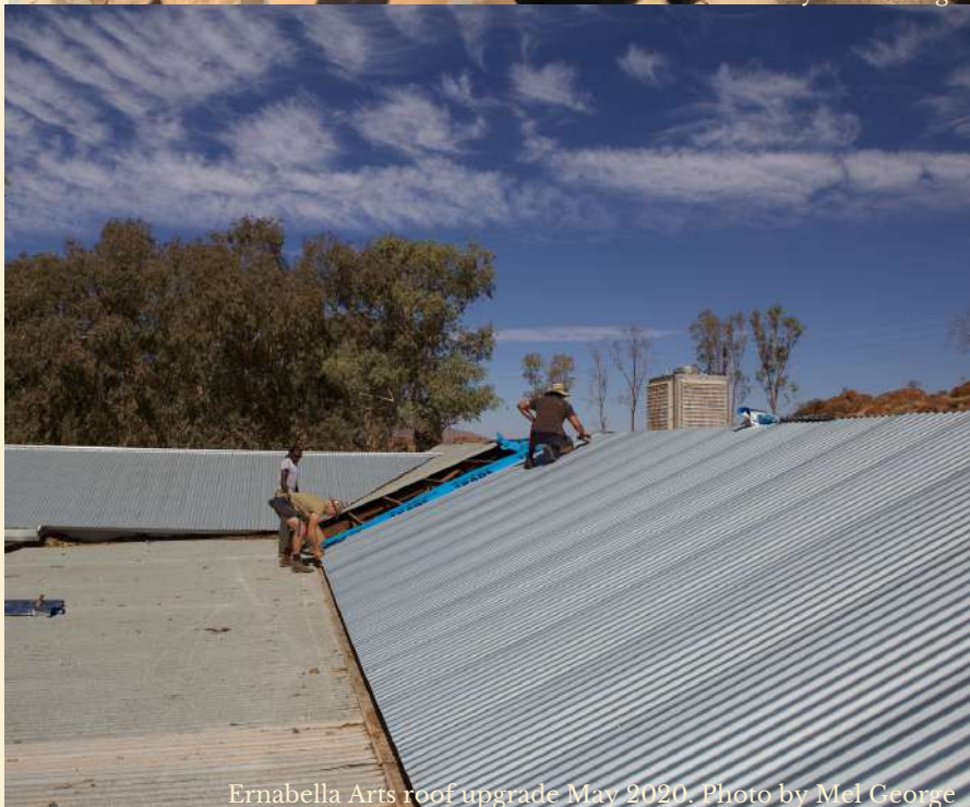
Murphy Goodwin working on Ernabella Arts roof upgrade May 2020 Photo by Mel George
